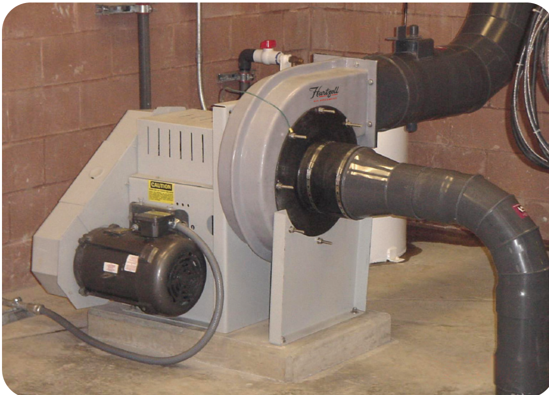
Series 43 Fiberglass Radial Blower at a Pump Station
