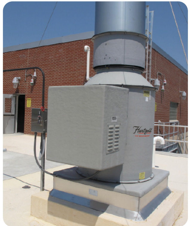
Series 40 Fiberglass In-Line Centrifugal Fan at a wastewater treatment plant.
